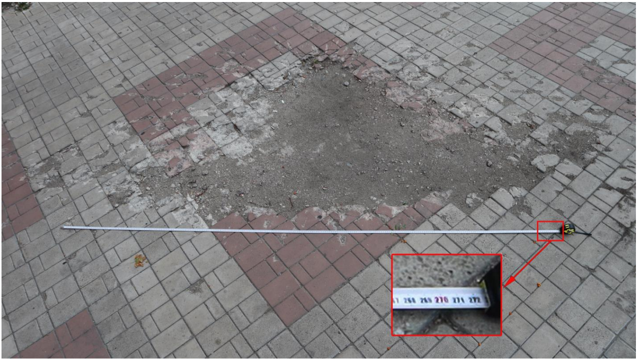
Fig. 8 – A crater in the cobblestone sidewalk next to the residential building at 59, Universitetskaya St.
