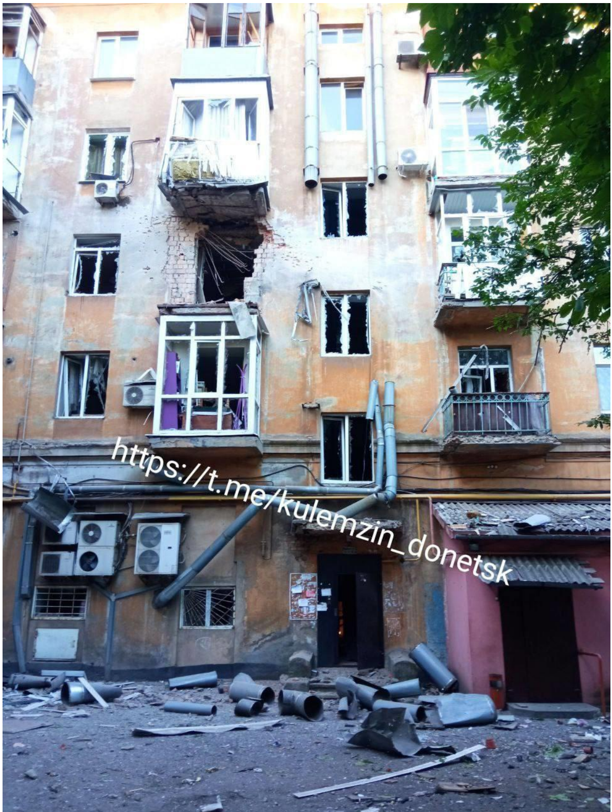
Fig. 17 – The result of a shell detonation in the wall of the residential building at 92, Artioma St. 28
