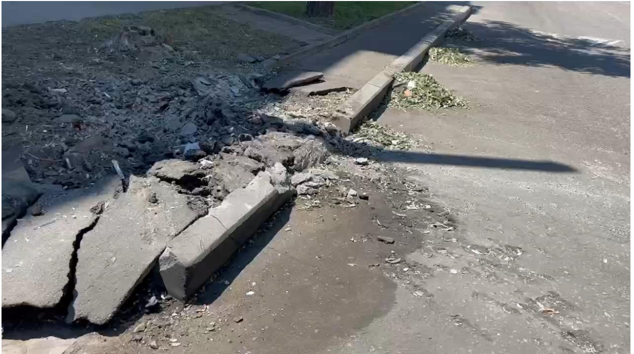
Fig. 6 - Consequences of a shell detonation in front of a building at 22, Vatutina St. 18
