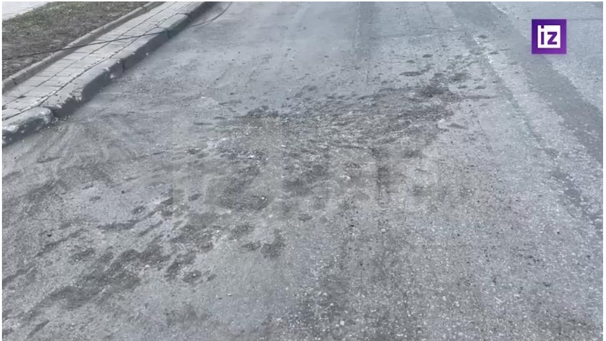
Fig. 10- A crater in the asphalt at the driveway between the Zvezdochka cinema and the residential building at 59, Universitetskaya St. 21
