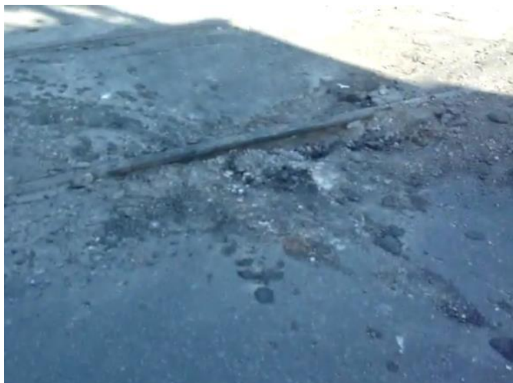
Figure 14. A crater from shell explosion on the tramway track opposite the residential building at 28, Gagarina St., Horlivka, 27.07.2014. 13
