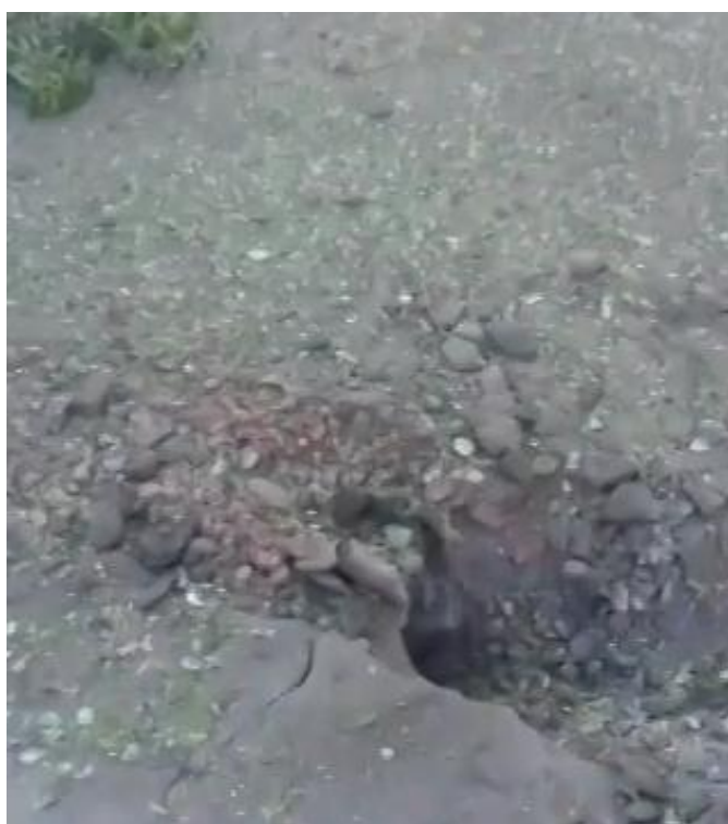
Figure 10. A crater in the road pavement next to School No. 85, Horlivka, 27.07.2014. 10
