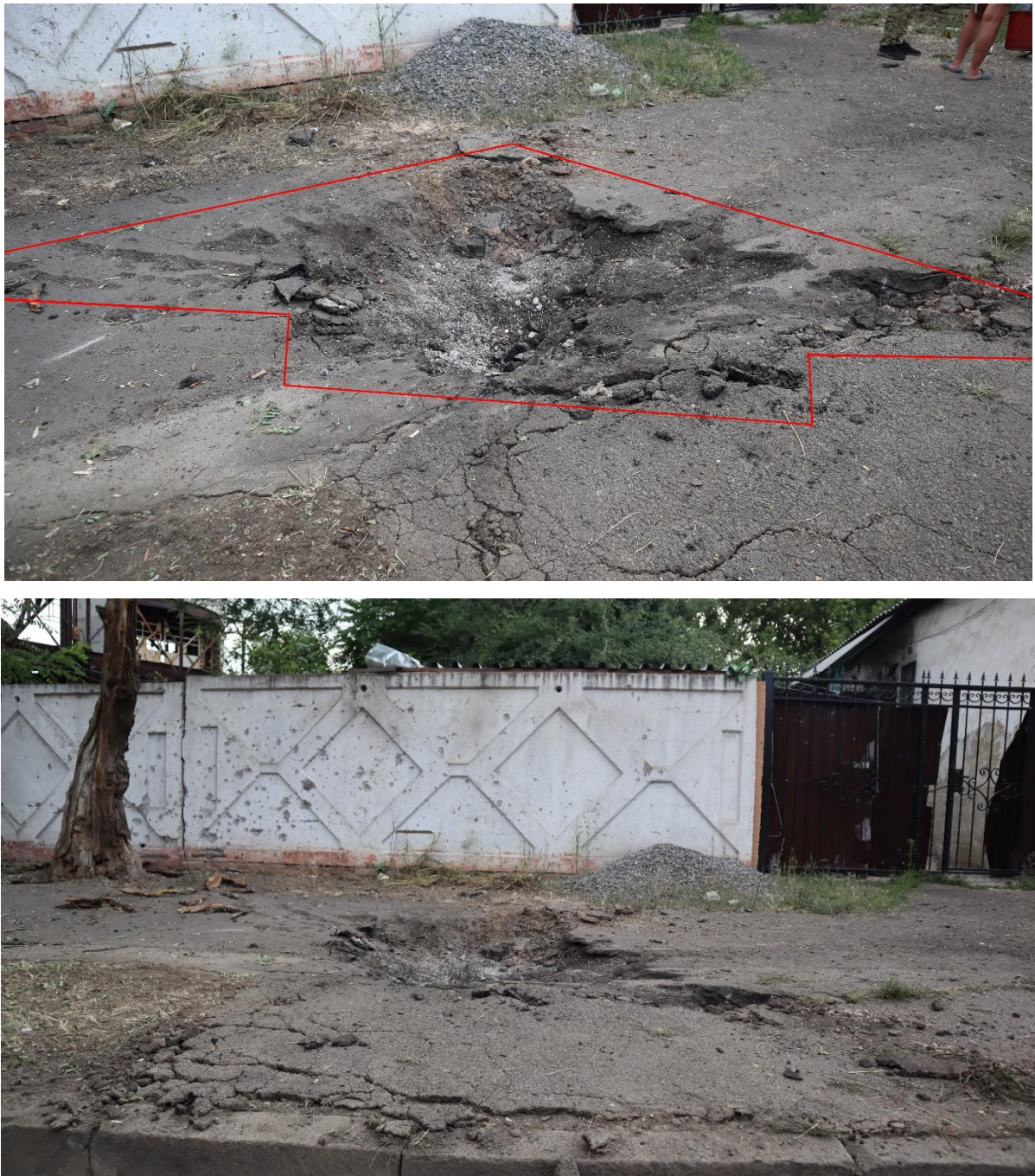
Fig. 3 - Consequences of a shell detonation near building No. 62 in Chelyuskintsev Street.
