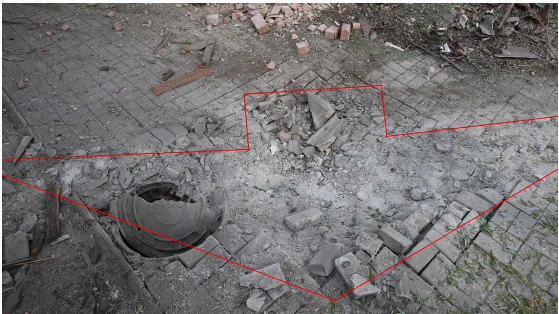
Fig. 4 - Consequences of a shell detonation near building No. 43 in Chelyuskintsev Street.
