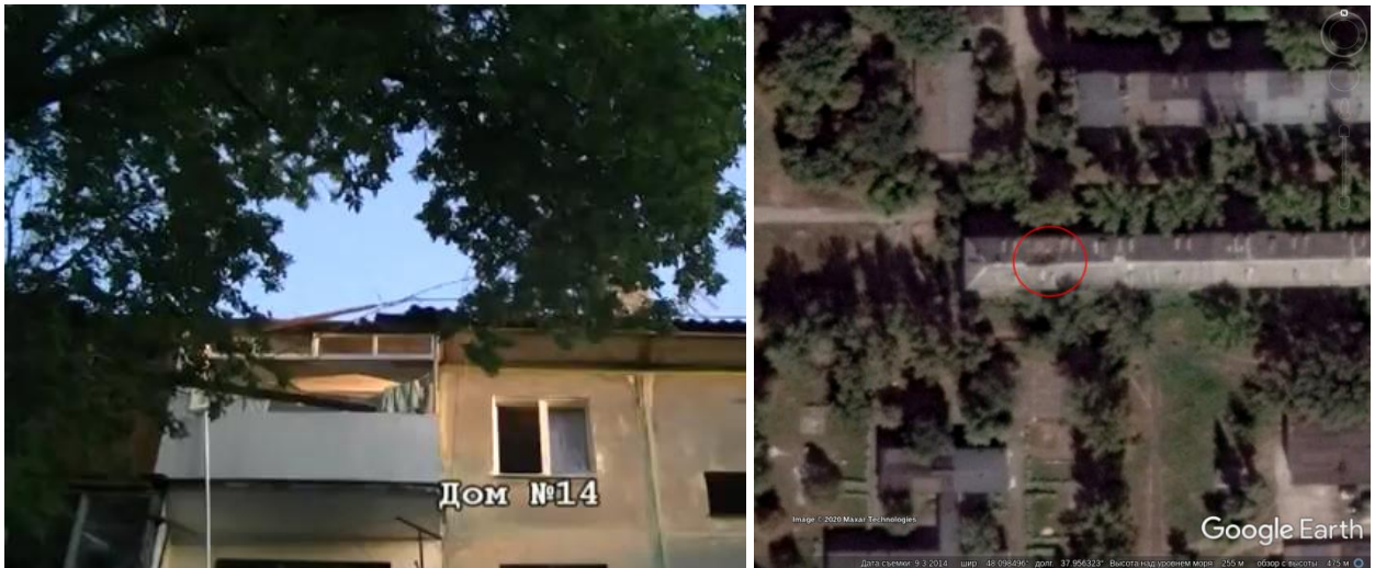
Fig. 4 - Shell hit (No.8) on the roof of the residential building at 14, Gvardeisky quarter: left — a screenshot from the video found on the Internet 6 ; right — a satellite image of 03.09.2014.
