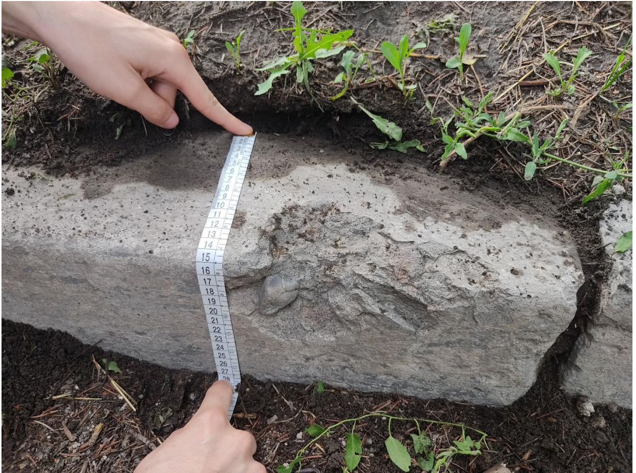
Fig. 21 - Measurement of the width and height of the visible part of the curb; to the right of the flexible tape - the same section of the curb damaged as a result of the shell explosion.
