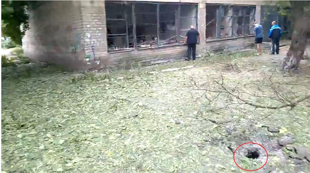
Fig. 8 - Shell hit (No.7) near the Northwest corner of the building of the Housing and Utility Management Office, Gvardeisky quarter 10 .
