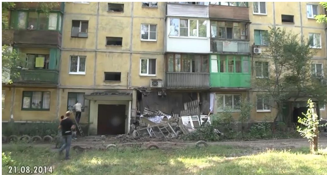
Fig. 11 - Shell hit (No.10) on the northern wall of the residential building at 13, Gvardeisky quarter at the ground floor level 13 .
