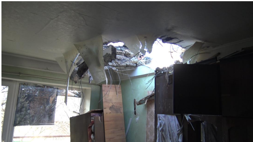
Fig. 8 - The hole in the ceiling of an apartment on the top floor of the residential building located at 15, Valeriya Arsenova St.
