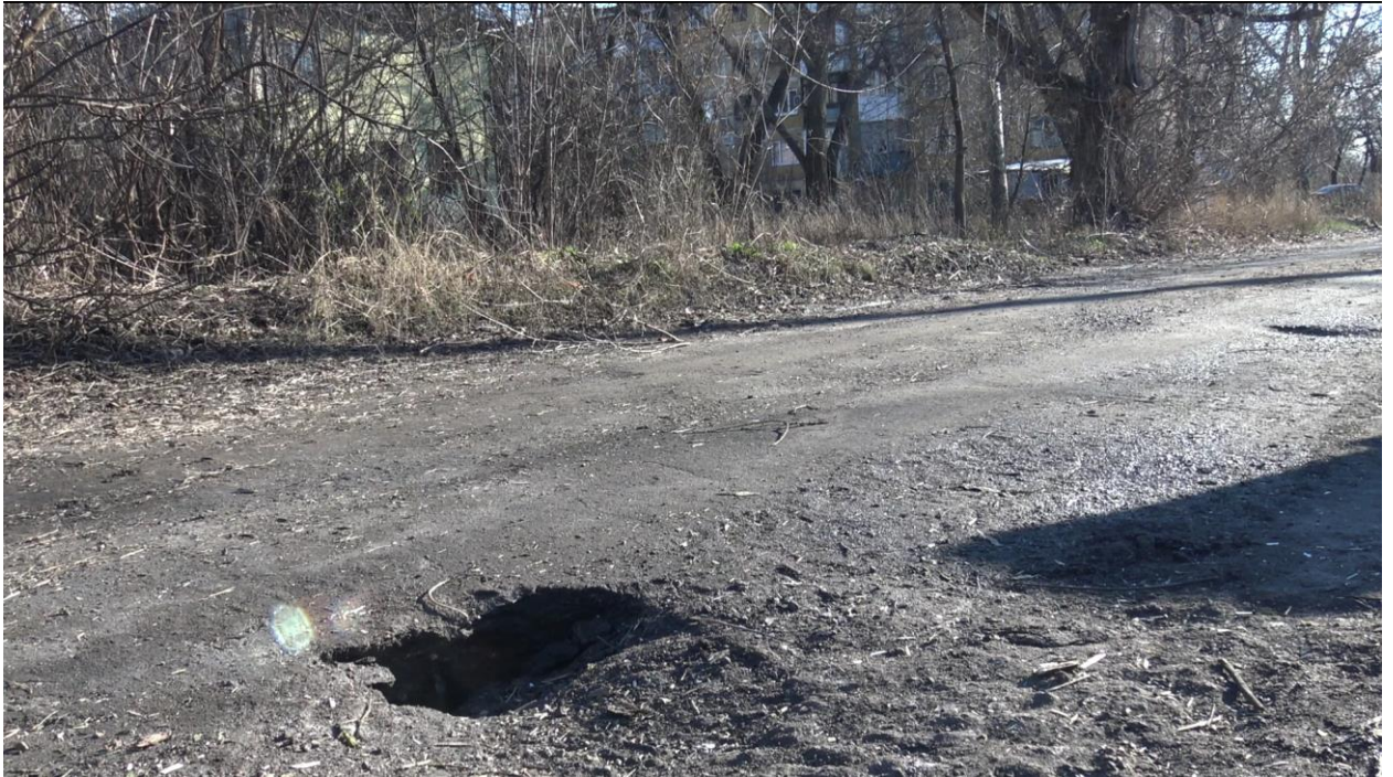
Fig. 9 - A crater on the asphalt road surface in Semionova-Tyan-Shanskogo St.
