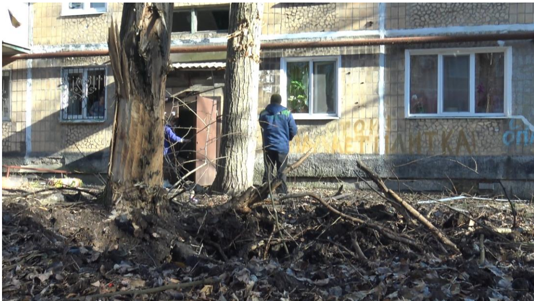
Fig. 5 - A crater caused by a rocket hit at the entrance to residential building at 22, Valeriya Arsenova St.
