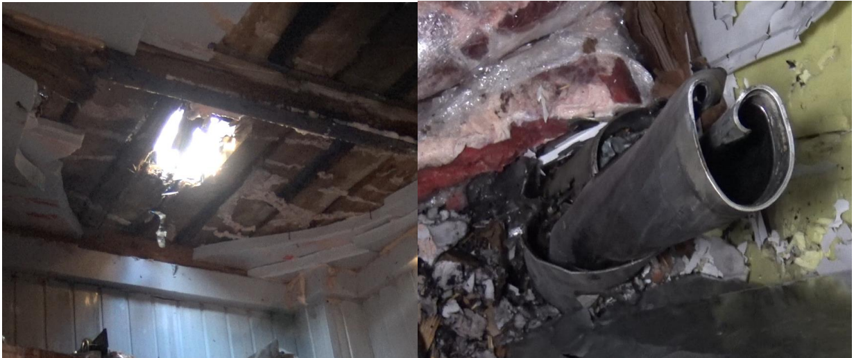
Fig. 2 - On the left - a hole punched by a rocket in the roof of the Petrovich food store; on the right - the remains of the rocket engine of an MLRS projectile in the warehouse of the Petrovich food store.
