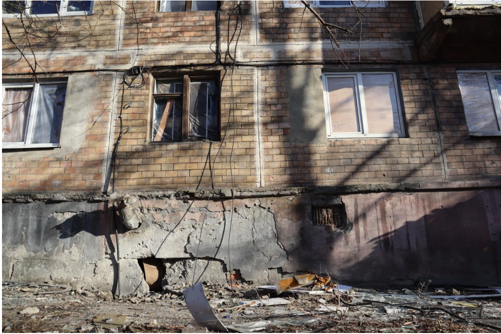
Fig. 7 – A hole on the wall of the residential building located at 19, Valeriya Arsenova St.
