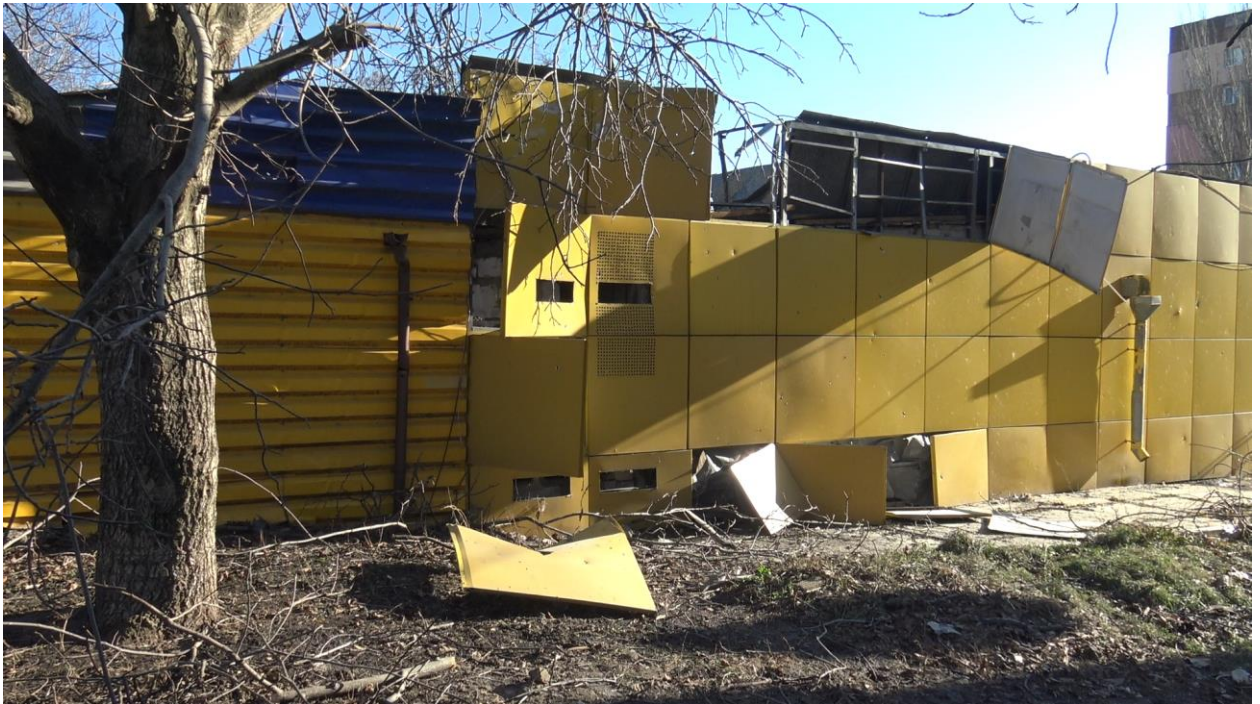
Fig. 3 - Destruction of the roof of the Petrovich food store, view from the street.
