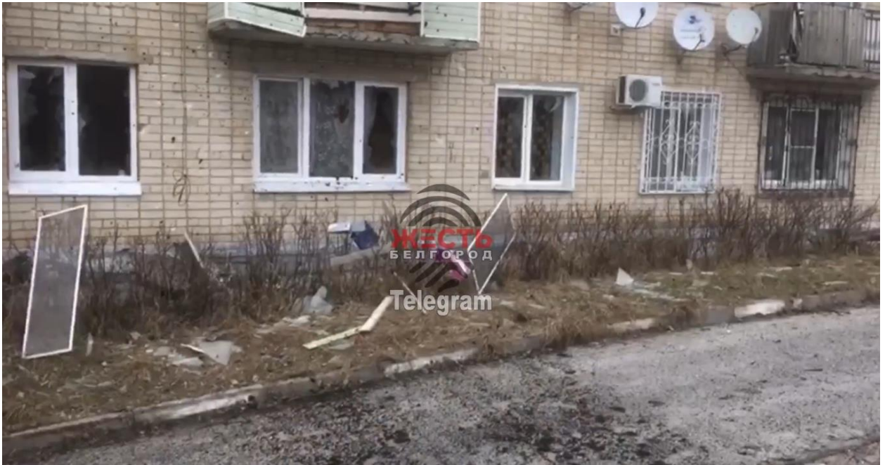
Fig. 4 – Consequences of an MLRS shell hitting the territory in front of a building at 2G, Gorkogo St.
