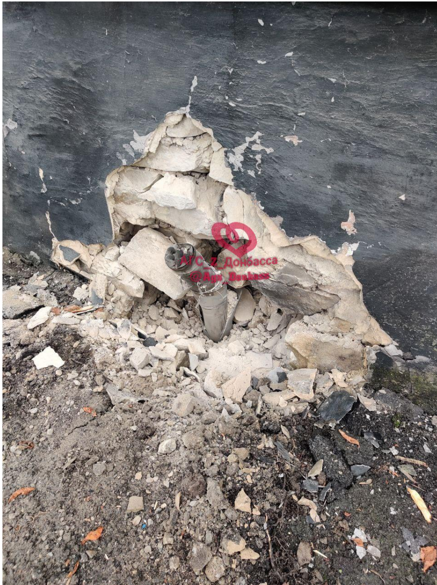
Fig. 4 – Shell hit in the multi-apartment residential building at 10, Donbass Liberation Str. 12 .
