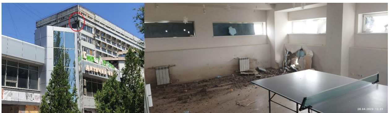
Fig. 25 – Shell hit on the building at 8B, Titova Avenue, (left photo: outside view, right photo 28 : inside view).
