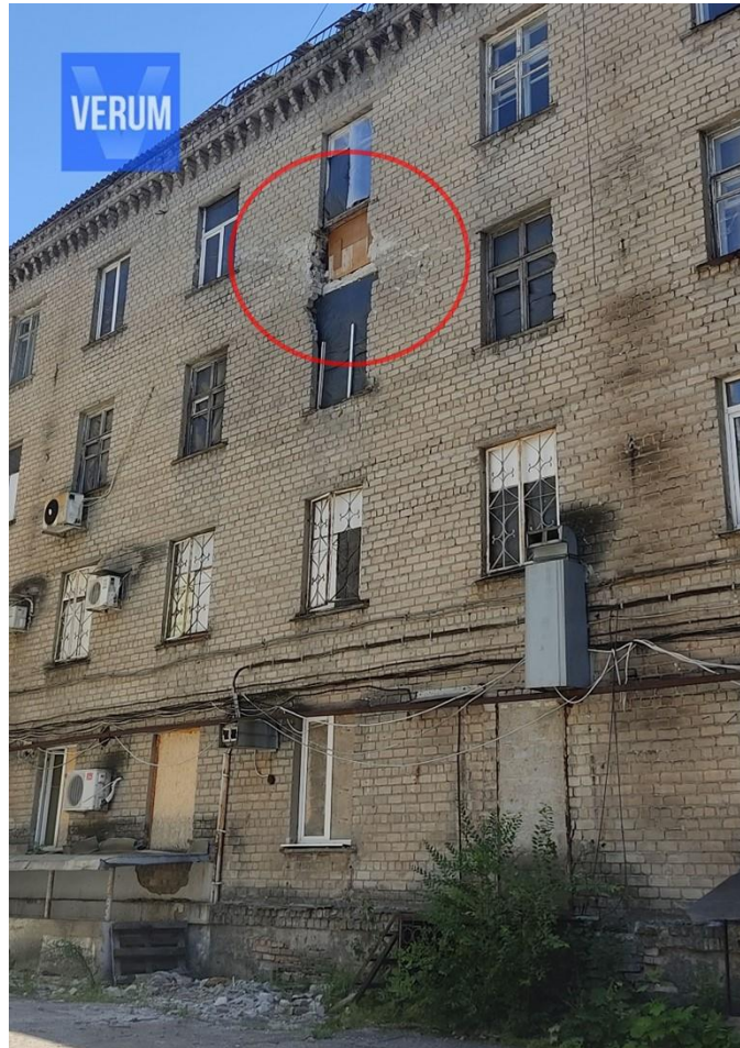
Fig. 11 – Shell hit in the building at 78, Universitetskaya St.
