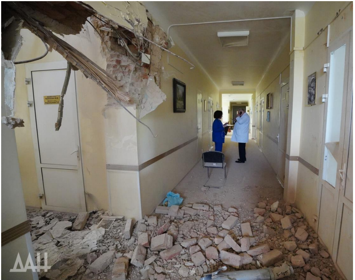
Fig. 19 – Consequences of the shell hit that damaged the main building of the Republican Traumatological Center 23 .
