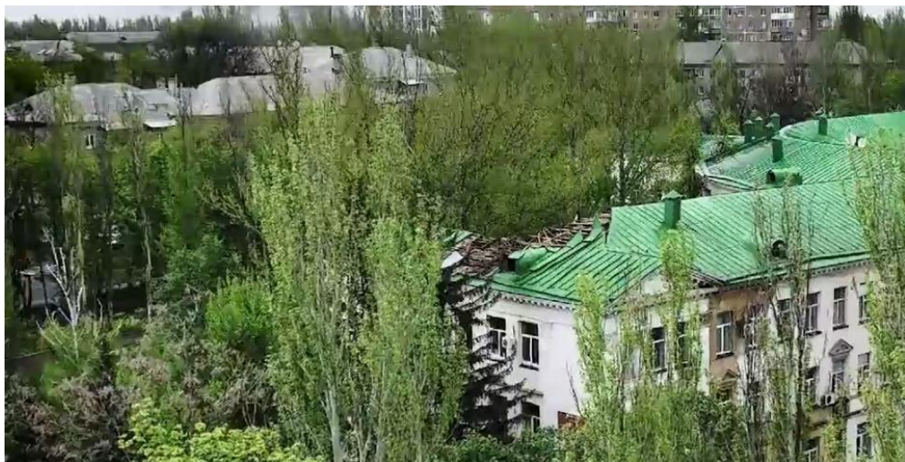
Fig. 18 – Shell hit on the roof of the Republican Traumatological Center 22 .
