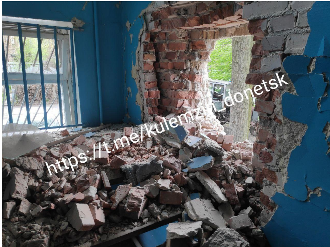
Fig. 5 – Shell hit in the building of the “Green Construction of the Kievskiy District” municipal enterprise at 102, Patrioticheskaya St. 13
