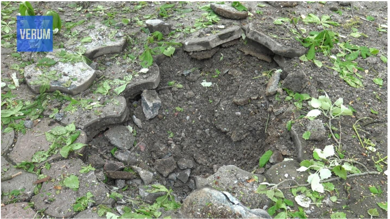
Fig. 8 – Shell hit in the paving slabs next to the residential building at 80E, Universitetskaya St.
