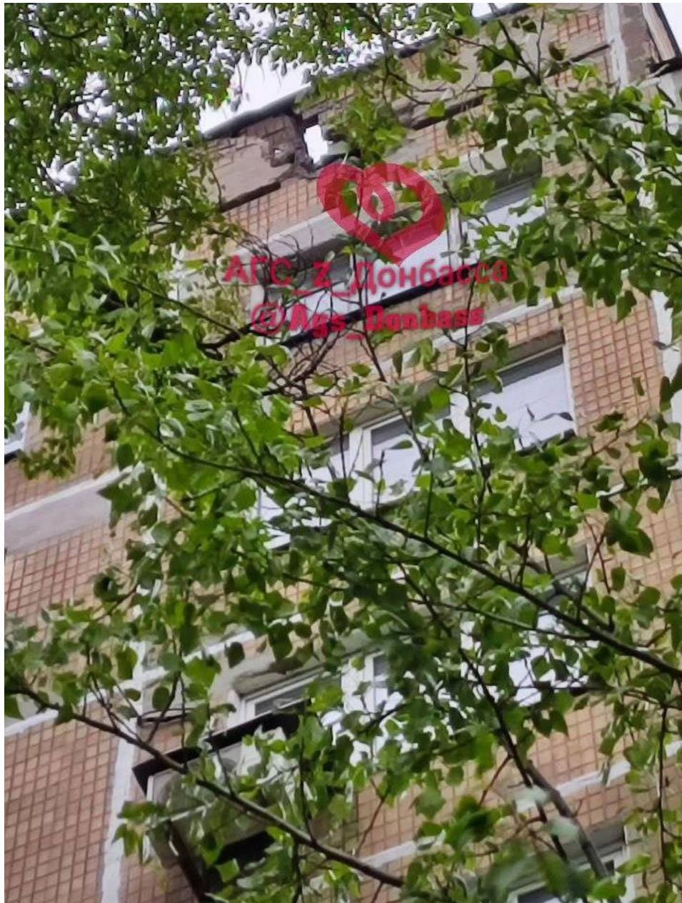
Fig. 13 – Shell hit on the multi-apartment residential building at 108A, Artyoma St. 19
