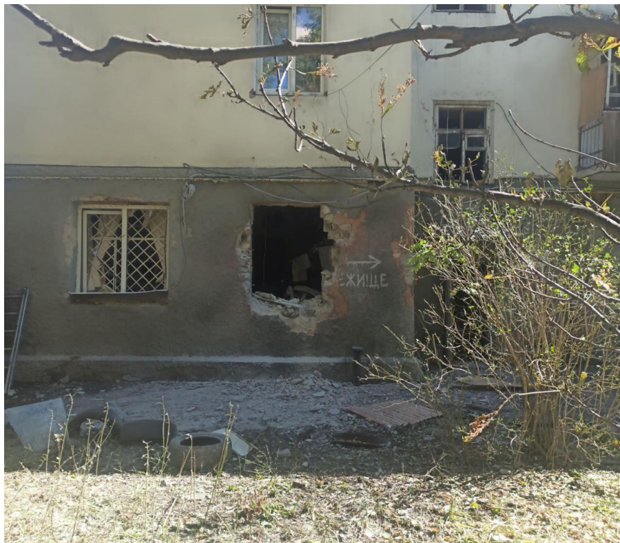
Fig. 3 – Detonation trace at the level of the ground floor window of the residential building at the address 1, Alexandr Matrosov Ave., Donetsk 34 .
