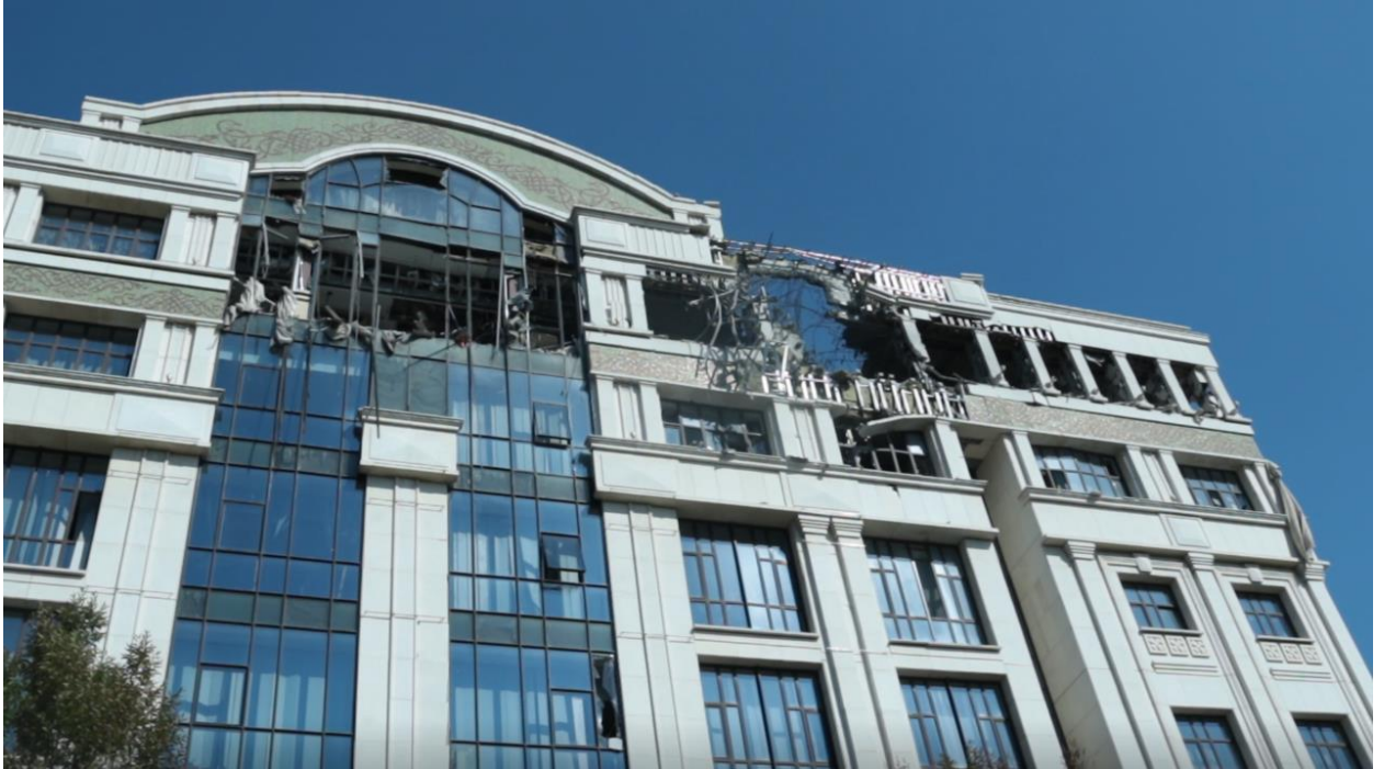
Fig. 9 – Destruction of the upper floor of the residential building at 7B Pushkina Blvd.
