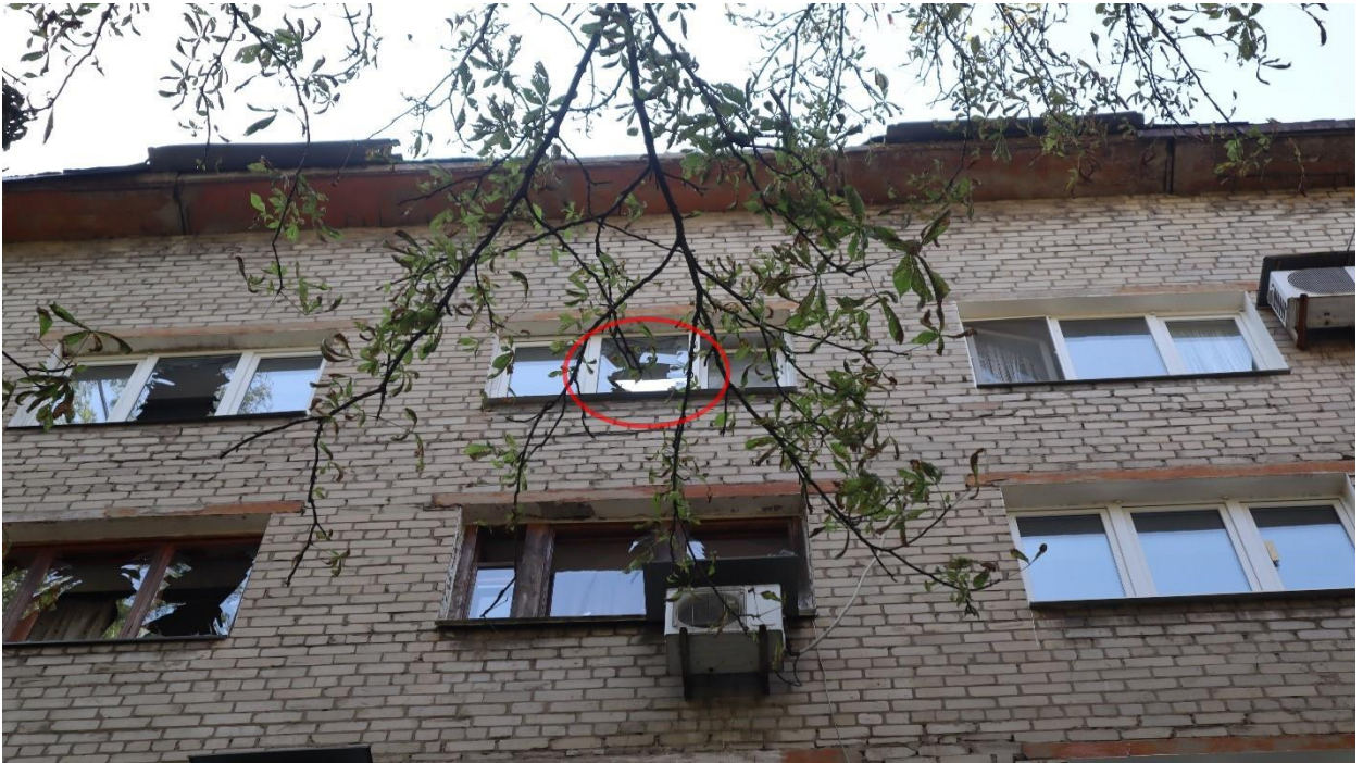
Fig. 2 – A hole in the roof at 4, Constitution Square.
