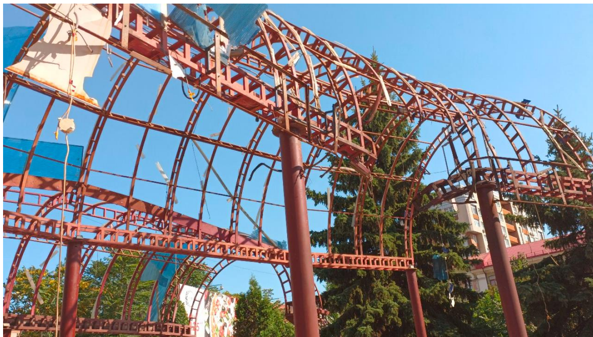
Fig. 7 – Damage to the entrance pavilion of the Central Hotel.
