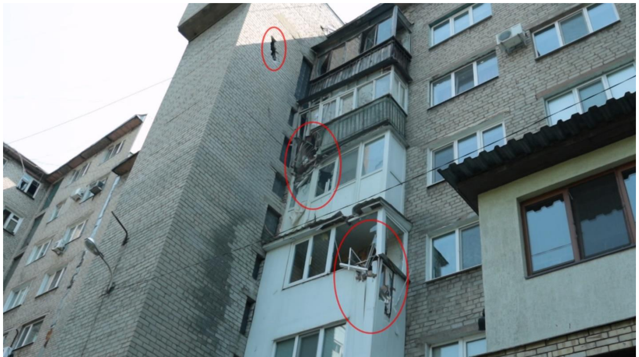
Fig. 3 – Damage to the wall of the residential building at 4, Constitution Square.
