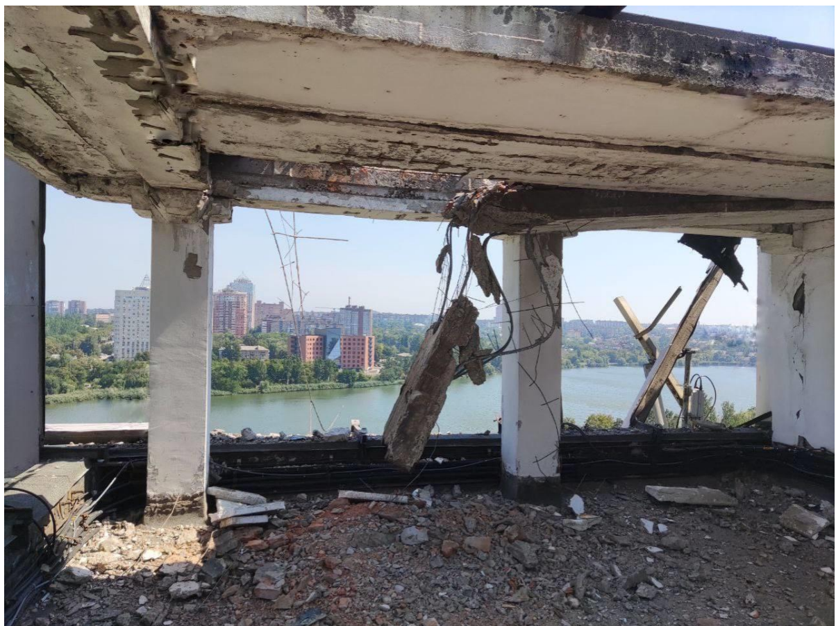
Fig. 6 – Damage to the roof of the “Kalmius” consumer services center 33 .
