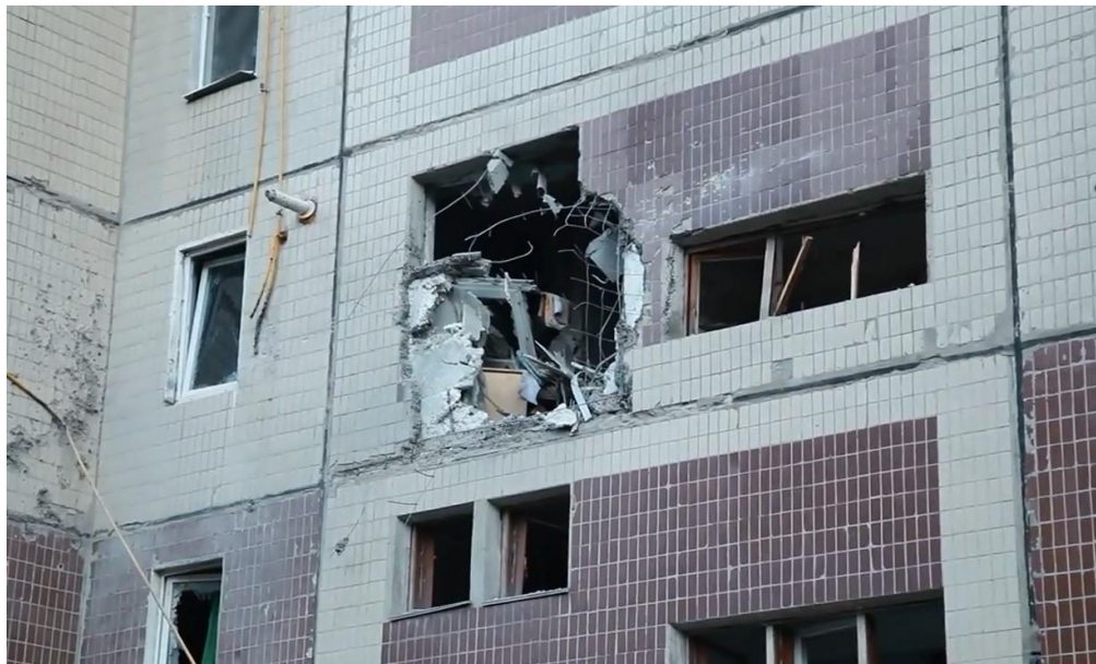
Fig. 9 – A hole formed as a result of the projectile-initiated detonation in the northern wall of a multi-storey residential building at the address 16, Olkhovsky quarter, Luhansk, at the second floor level 21 .
