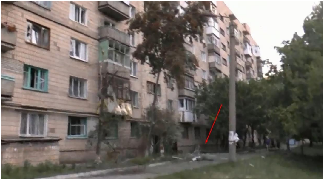
Fig. 16 – A crater in the yard of a multi-storey residential building at 79A, Andrey Linyov St., Luhansk, between 1 and 2 entrance halls 28 .
