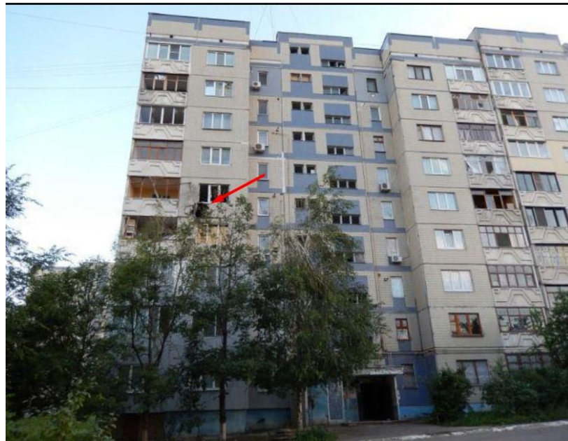
Fig. 8 - A shell hit on the northern wall of a multi-storey residential building at the address 6, Stepnoy quarter, Luhansk, at the fourth-floor level 20 .
