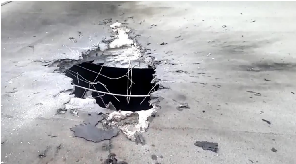
Fig. 27 – A hole broken by a projectile in the roof of the utility premises located to the north of the building at the address 75 lit. Z, Andrey Linyov St., Luhansk 38 .
