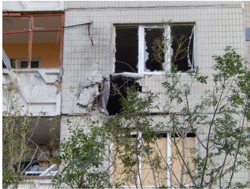
Fig. 7 – A shell hit on the northern wall of a multi-storey residential building at the address 6, Stepnoy quarter, Luhansk, at the fourth-floor level 19 .
