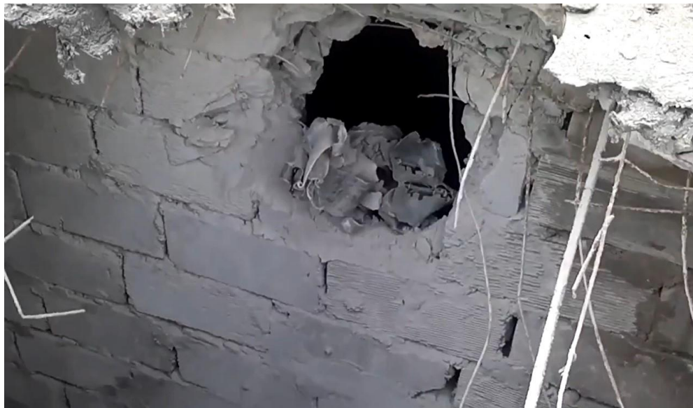
Fig. 26 – A hole cut off as a result of the projectile detonation in the inner wall of the utility premises located to the north of the building at the address 75 lit Z, Andrey Linyov, Luhansk 37 .
