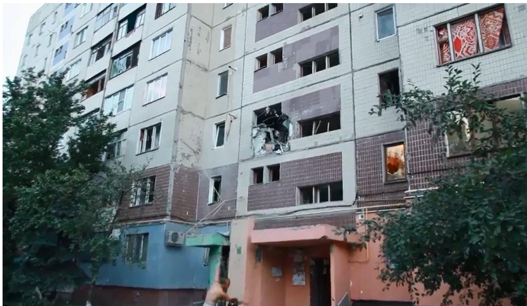
Fig. 10 - A hole formed as a result of the projectile-initiated detonation in the northern wall of a multi-storey residential building at the address 16, Olkhovsky quarter, Luhansk, at the second floor level 22
