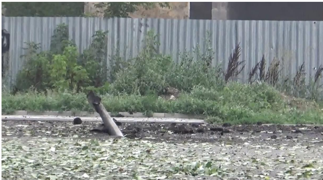
Fig. 12 - Debris of the projectile missile part in the road pavement at the exit from Andrey Linyov Street, opposite the western end of the residential building at 79A, Andrey Linyov St, Luhansk 24 .
