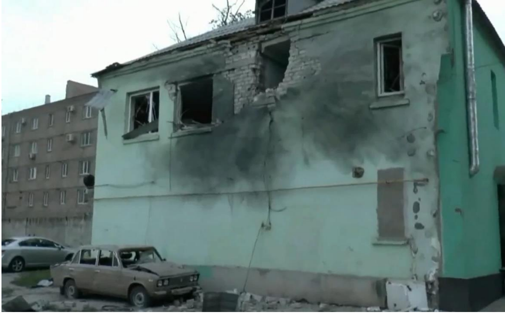
Fig. 17 – A hole formed as a result of the projectile-initiated detonation in the northern wall of the two-storey residential building at 75L, Andrey Linyov St., Luhansk, at the level of the 1st floor. 29
