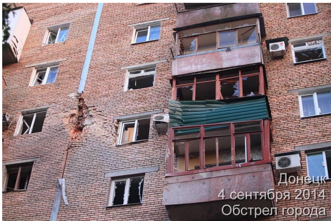
Fig. 9 – Shell hit No. 12: 13, Kutuzov St. 27
