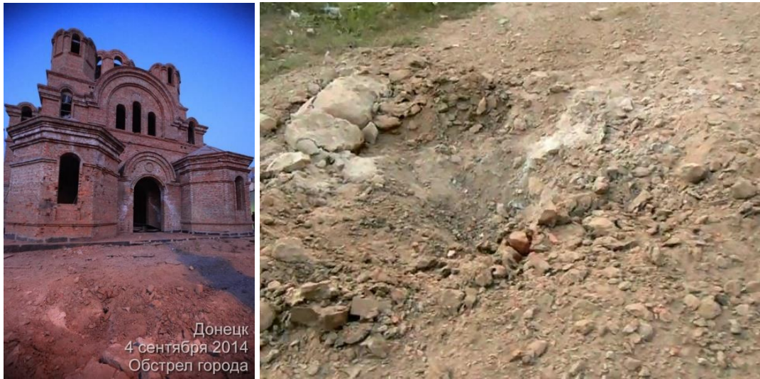
Fig. 25 – Shell hit No. 19: Temple of the Holy Great Martyr Panteleimon the Healer. On the left: a crater from the projectile and damage on the wall of the temple 39 ; on the right: crater enlarged view 40 .
