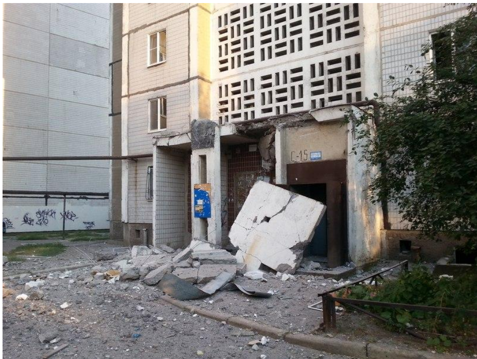
Fig. 13 - Piece of concrete slab that fell on the driveway in shell hit No. 13 31 .
