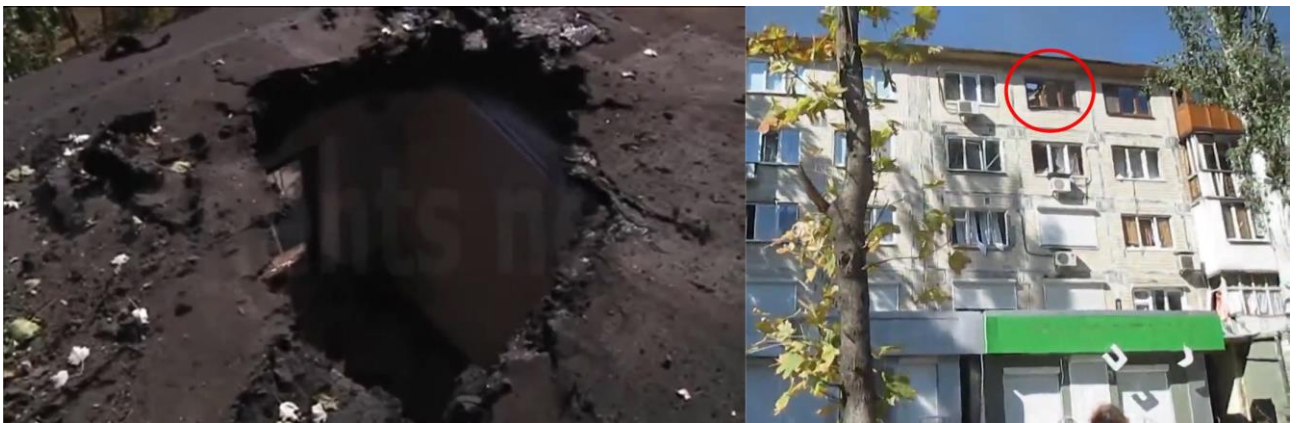
Fig. 9 – The trace of projectile hitting in the roof of the multi-storey residential building at 56, Shevchenko Blvd. (left: view from the building roof 37 ; right: view from the roadway in Shevchenko Blvd 38 ).
