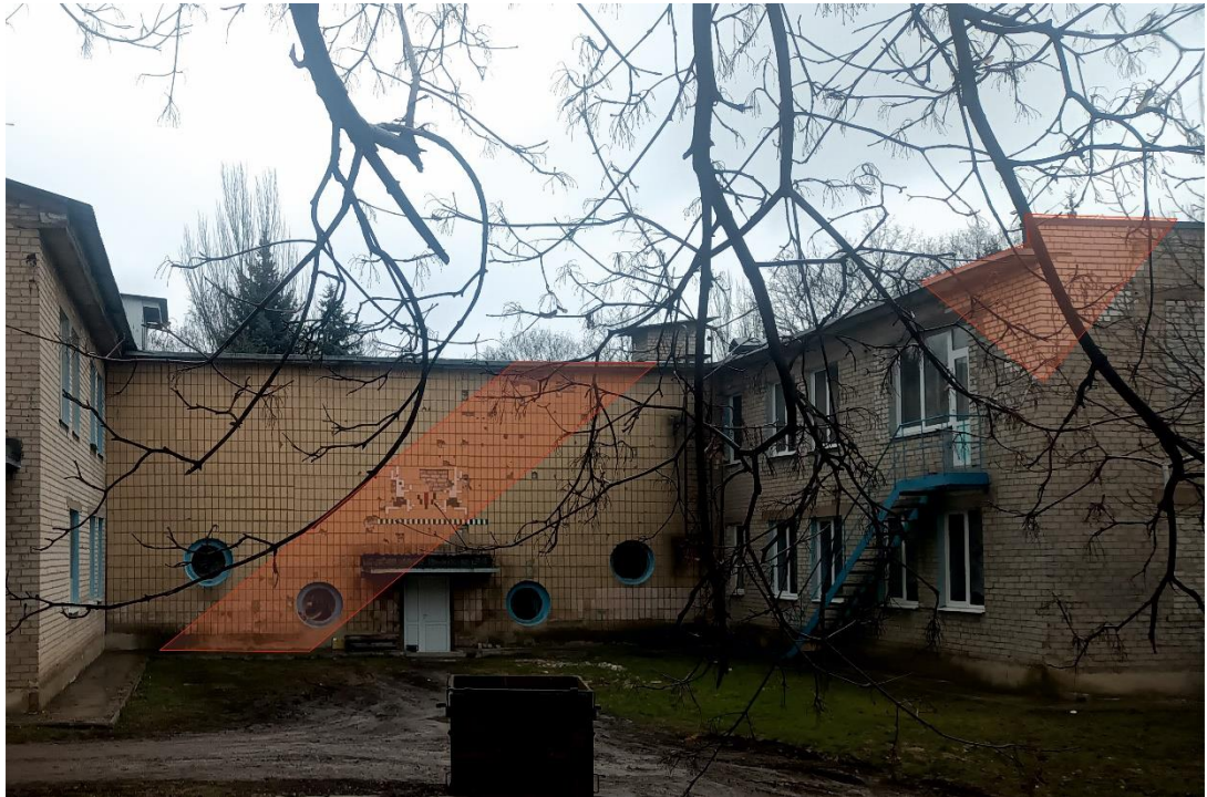
Fig. 28 – Traces from the main scatter of fragments on the wall to the north-east of shell hit 2 (photo from February 12, 2022).
