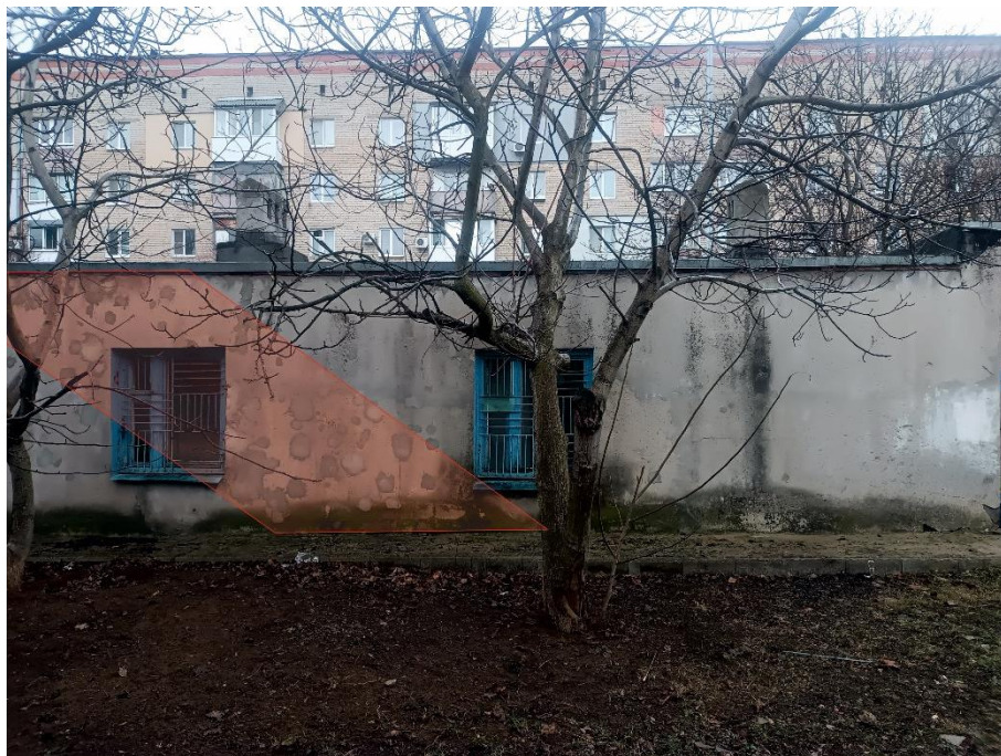
Fig. 27 – Traces from the main scatter of fragments on the wall to the south-west of shell hit 2 (photo dated February 12, 2022).
