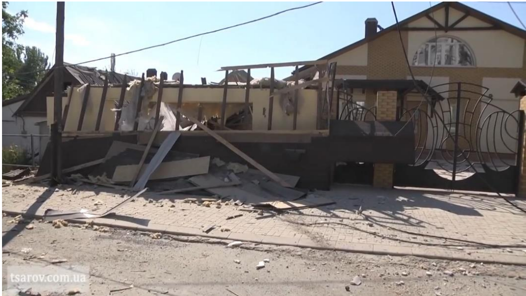
Fig. 2 – Consequences of shell hitting the territory of a private household at 49, Lazarenko St. 33 .
