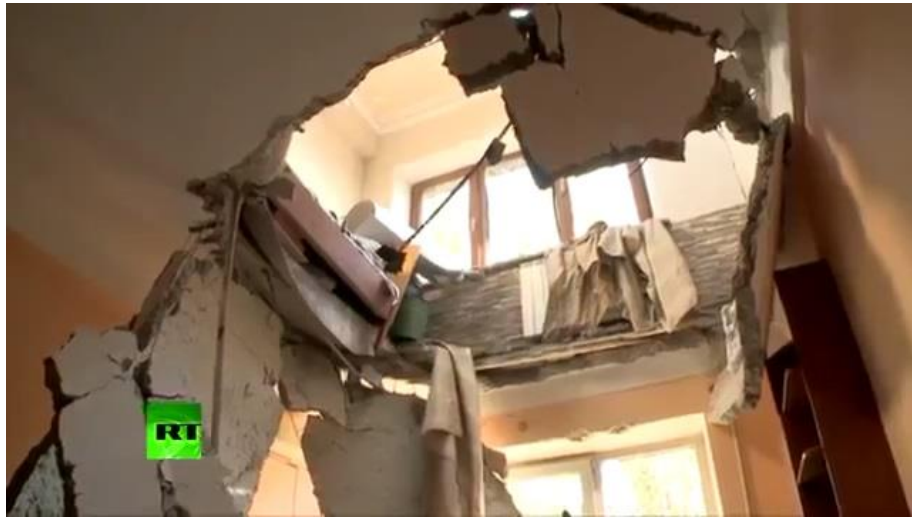
Fig. 10 – Consequences of projectile hitting in a multi-storey residential building at 56, Shevchenko Blvd. 39
