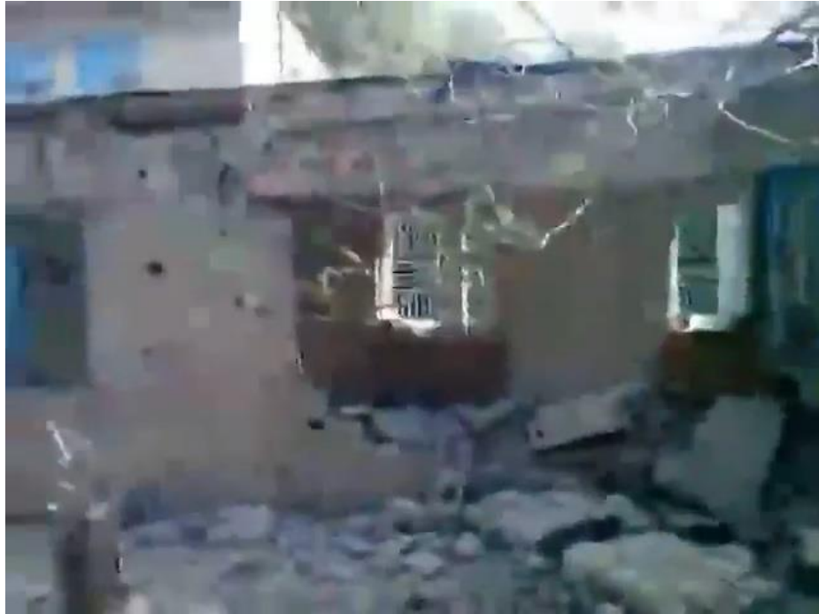
Fig. 6 – Significantly damaged passage between the building of the educational complex No. 16 and the garages at 66A, Shevchenko Blvd. 35
