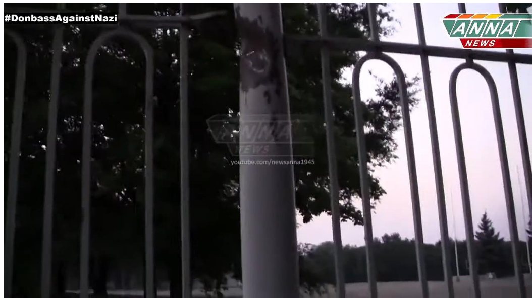
Fig. 21 – Damaged fence 40 meters north of the Palace of Youth located at 189, Chelyuskintsev Str. 39 .
