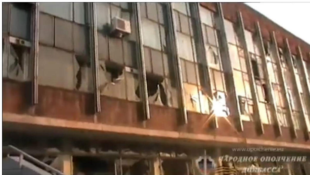
Fig. 20 – Damaged glazing of the building of the Youth Palace, which is located at 189, Chelyuskintsev St. 38 .
