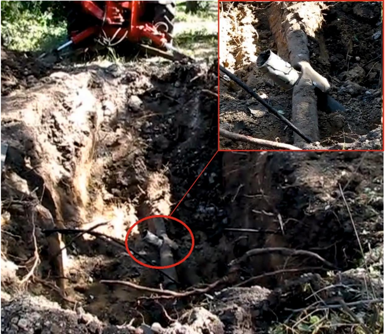
Fig. 12 – Debris of the MLRS projectile MP in an underground gas pipeline 5 meters away from a private house at 70, Baidukov St 30 .
