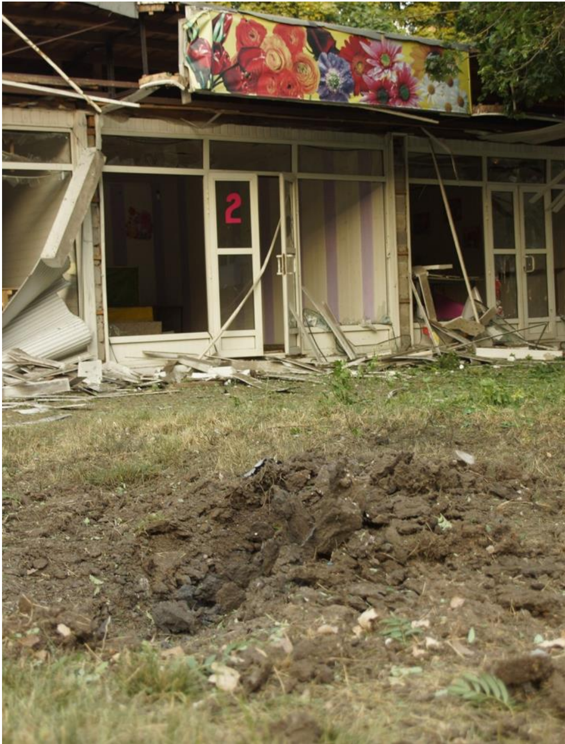
Fig. 16 – The shell hit in the ground surface, a few meters west of the pavilions selling flowers at 189A/1, Chelyuskintsev St 34 .
