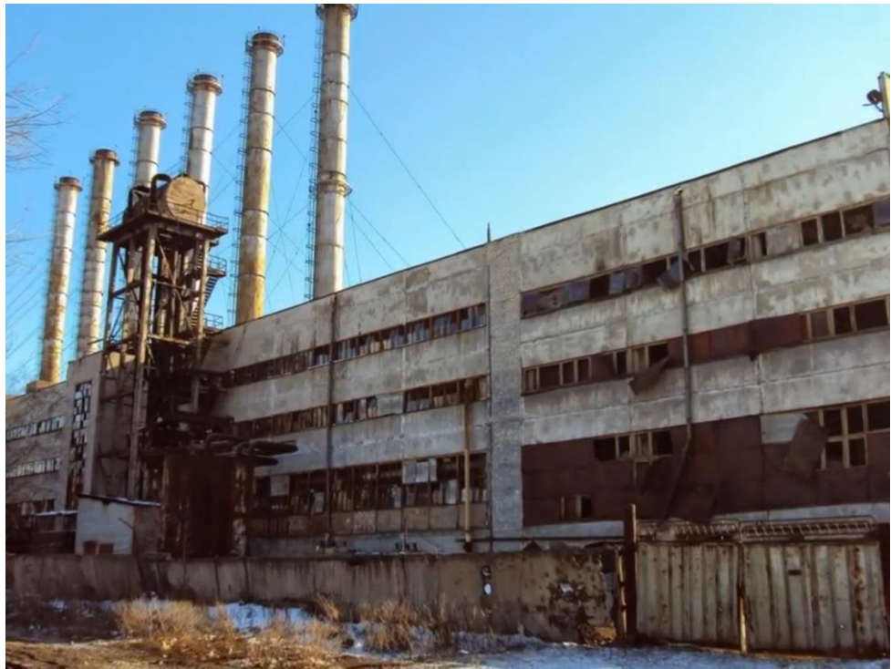
Fig. 6 – The building of the municipal boiler station damaged by shell hit 3 35 .
