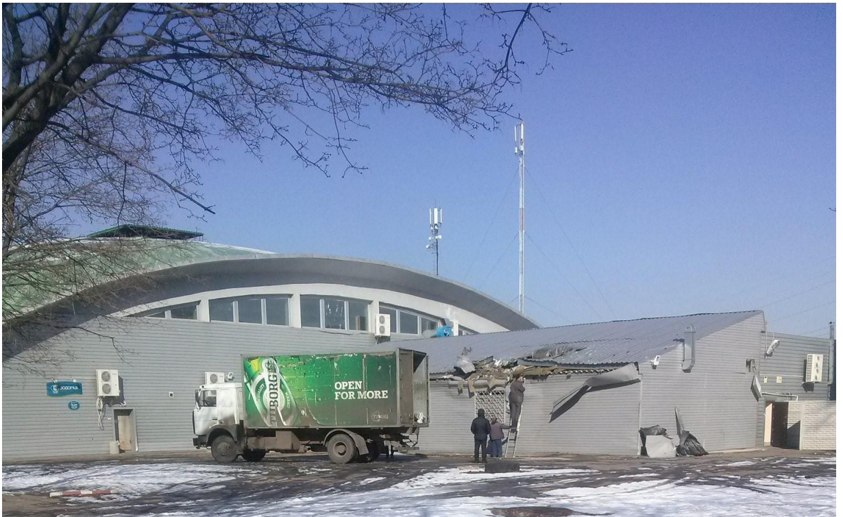
Fig. 19 – Part of the roof damaged by shell hit 13 48 .
