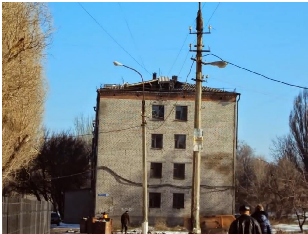
Fig. 7 – The roof of the building damaged by shell hit 5 36 .
